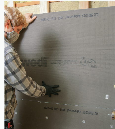
Add wall panels. Start from the bottom and work upward. Wall panels get a bead of sealant in the joints also.
