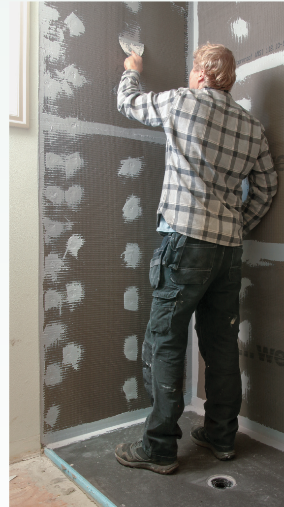
Done in a day. Seal every screw and plumbing penetration with the Wedi sealant, leave it 20 to 30 minutes to skin over, and you're ready for tile.
