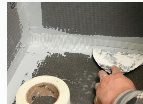
Tape adds insurance. For added resistance to movement in the framing and substrate, I add fiberglass tape at the joints around the shower pan, embedding it in the sealant.
