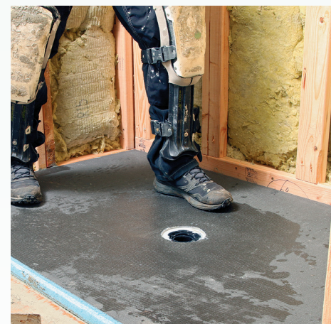
Place the pan. Walk all over the pan to collapse the thinset ridges and ensure the pan is fully bonded.
