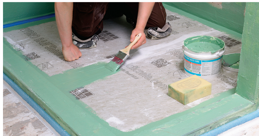
Coat the seams. Though not specifically required by this system, liquid-applied waterproofing is cheap insurance, and every brand offers it. The shower curbs are formed with cement backerboard and covered with the bonded sheet membrane before I brush on the liquid-applied product.
