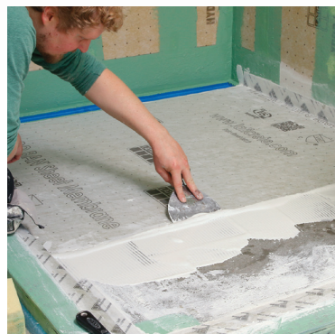
Sheet membrane is last. Finally, I apply a sheet membrane over the mud-bed shower pan, letting the banding set up for an hour or two before applying the main sheet. I wait so the banding won't slide when I bed and smooth the final layer in thinset.
