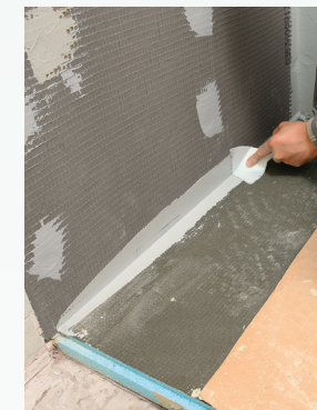
More sealant over the seams. A bead of sealant goes over every seam and is troweled flat.
