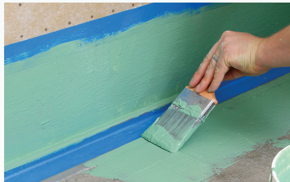
Liquid-applied membrane is a versatile tool. After finishing the mud-bed pan, I waterproof the drain area with two coats of a quick-curing liquid membrane from Laticrete, building a seal 6 in. up and out in all directions.
