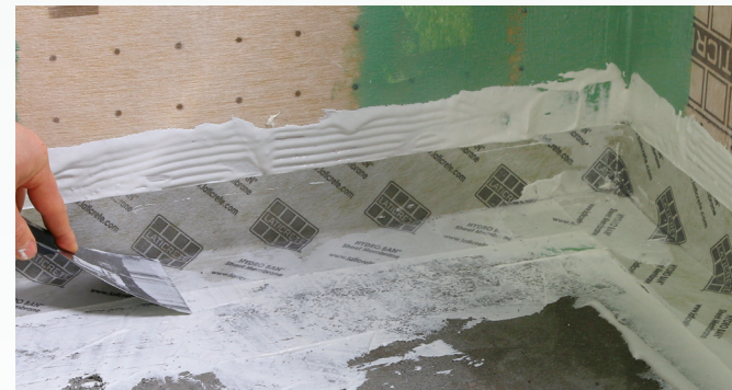
Fabric banding at the edges. To prevent cracks in the tile and grout, the critical joints around the pan get a fabric banding. Like the liquid membrane, this is designed to go over damp concrete for the best bond, so you might have to dampen the mud bed before installing it.
