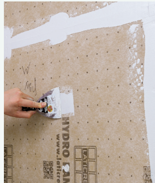
Walls are easy. Foamboard cuts with a utility knife and attaches with specialized screws. Run a bead of sealant between each panel and trowel more over the seams, then coat fasteners and seal around penetrations.
